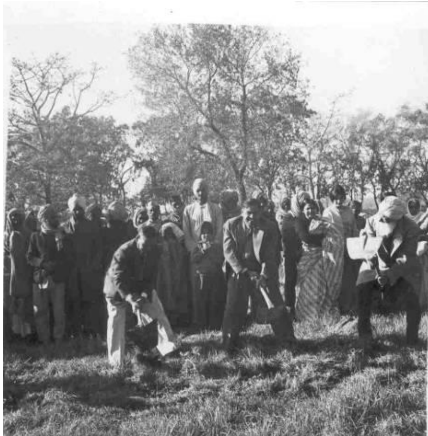
Digging for Gold? Mr Kate makes the first dig for the Swimming Pool. Among the onlookers at the back is Miss Lila Bhan Kak on the right.
